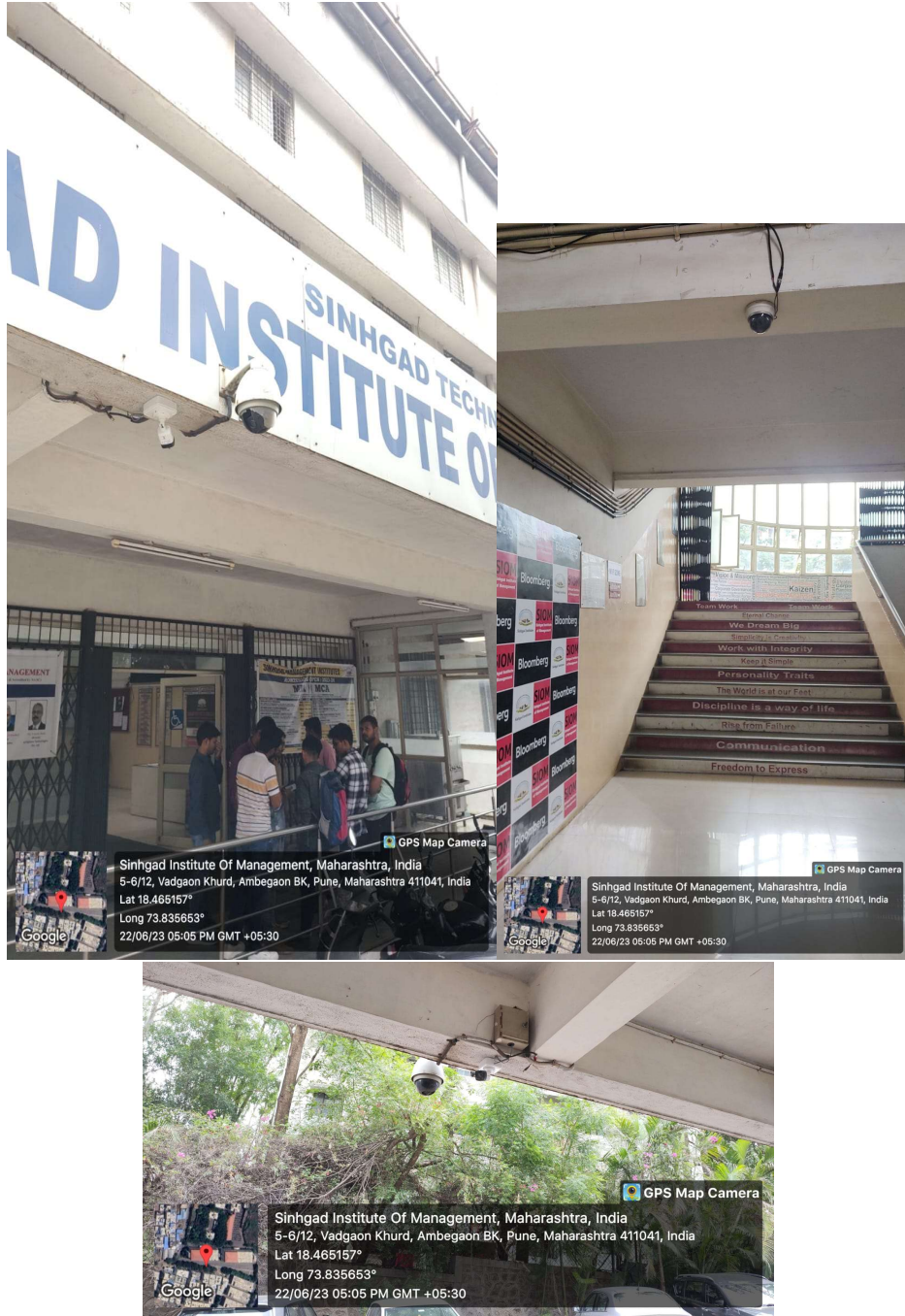
Security Cameras Inside Campus Building
