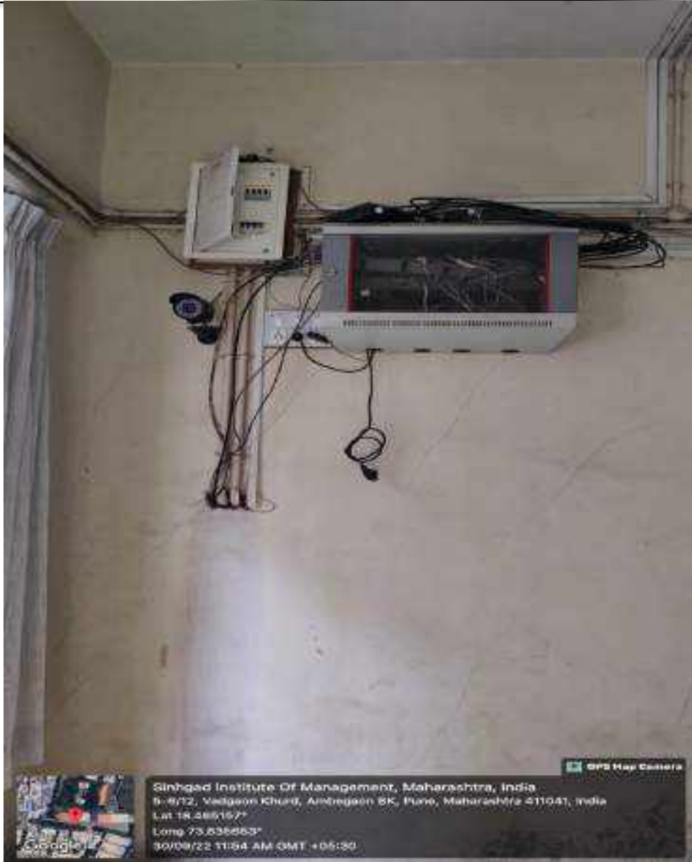
Central Library – Internet Switch
